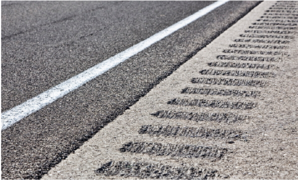
Edgeline rumble strips.
